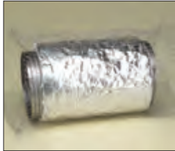
...which slips around the insulated liner. Try pre-rolling mesh like a nylon stocking, then unrolling around liner.
